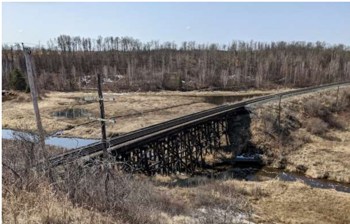
One of the many wooden trestles on CN's Edmonton – Calgary line within the city limits of Camrose (Doug Burton photo)
